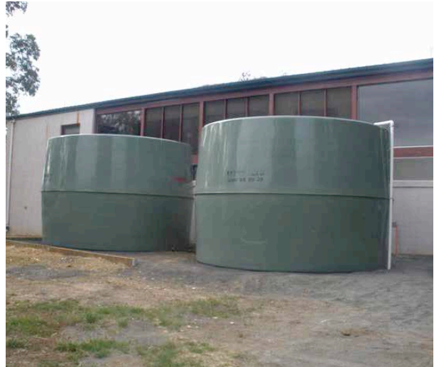
Installed water tanks at the Creswick facility
